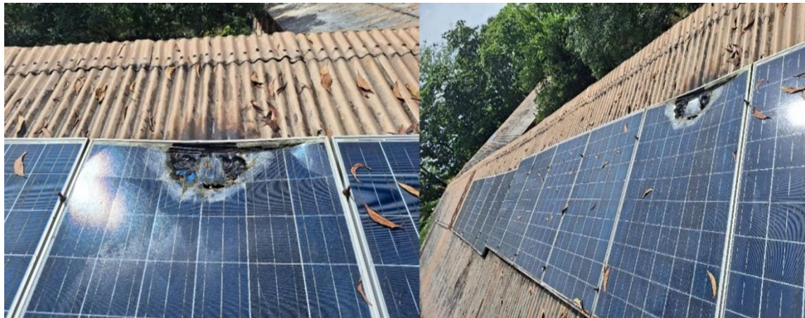
Figure F1. Photographic display of the destruction of solar panels caused by thunder in October 2023
