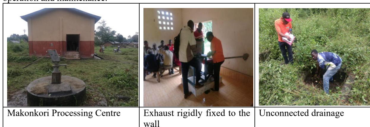
Figure B11. Faulty exhaust and drainage pipe connection
